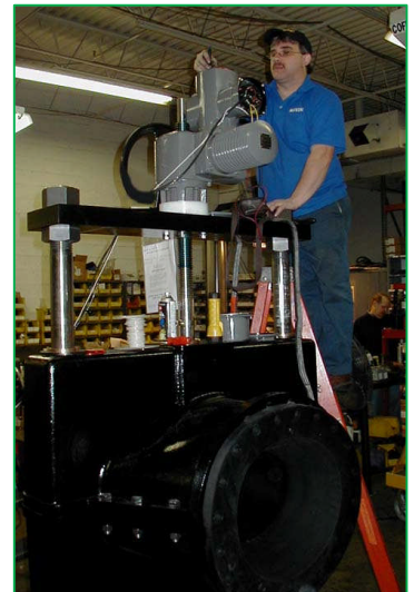
Electric Actuator on 20" valve
